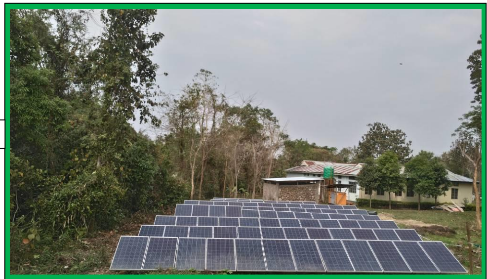
Solar Power Plant
